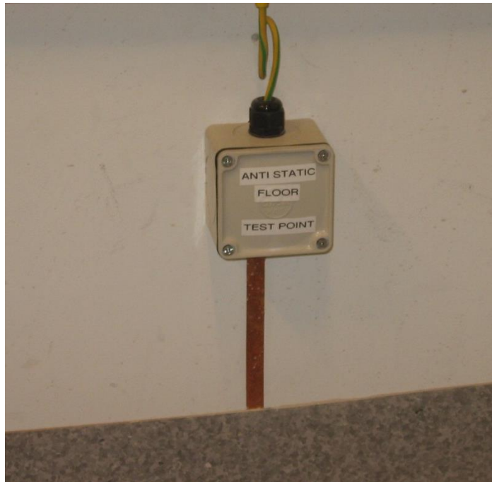
Figure 7.7 — Typical Antistatic Flooring Junction Box
