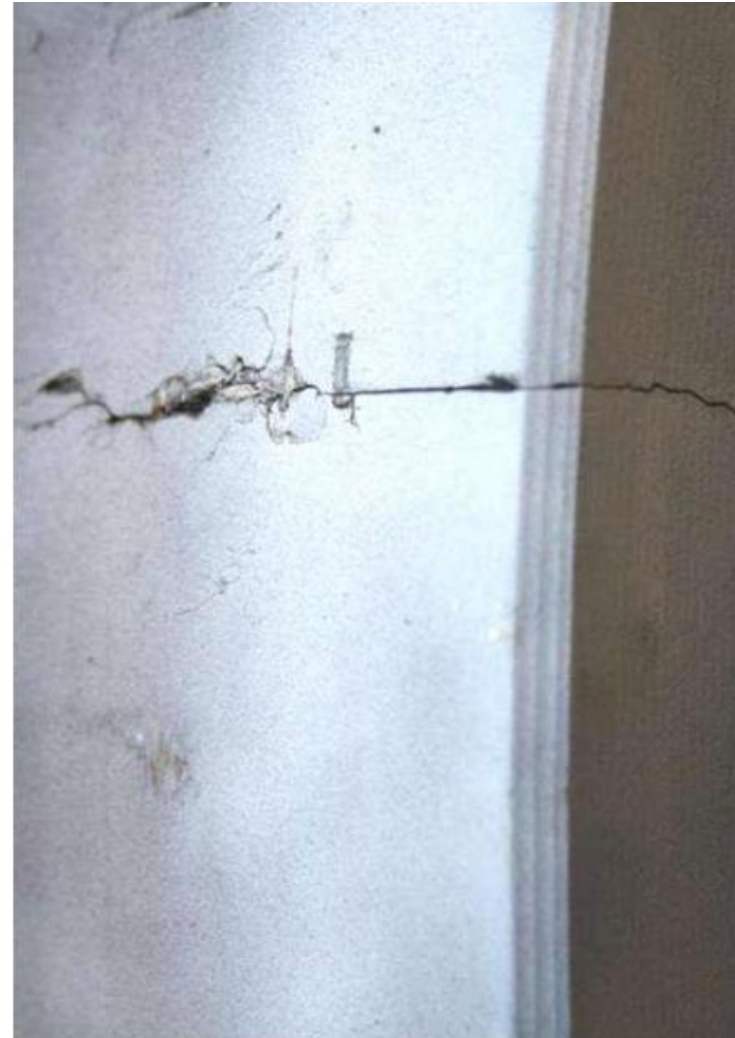
Figure 29 – Class 5 Thermal Crack
