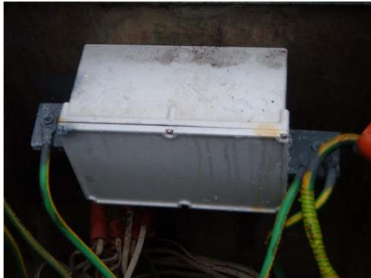
Figure 14.9.4.1 – Earthing Diode Assembly External View
