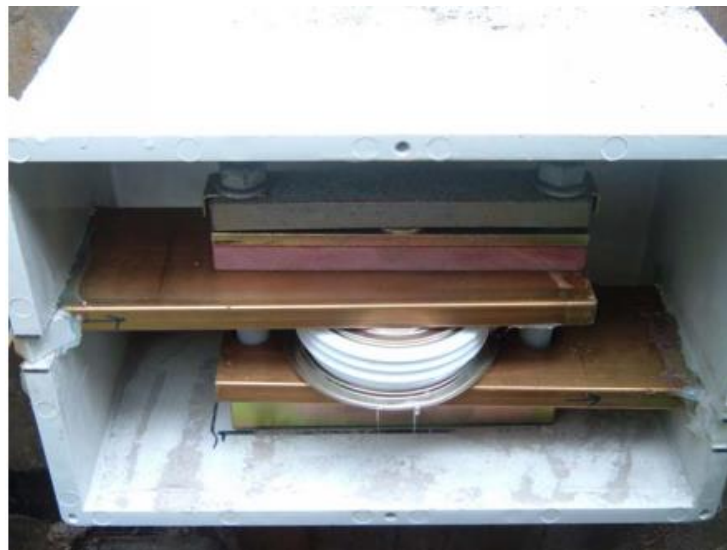
Figure 14.9.4.2 – Earthing Diode Assembly Internal View
